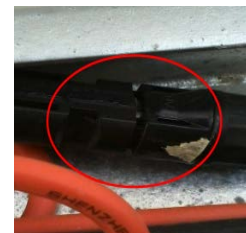
The cable is loose
